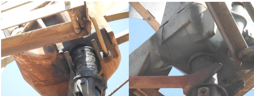
*Broken spiral at Charleville common bore & cracked casting at YoYo mill
