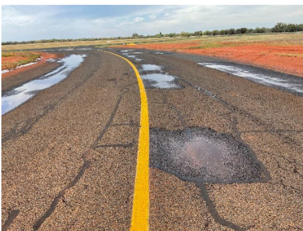
Taxi way – ponding of water – Charleville Airport
