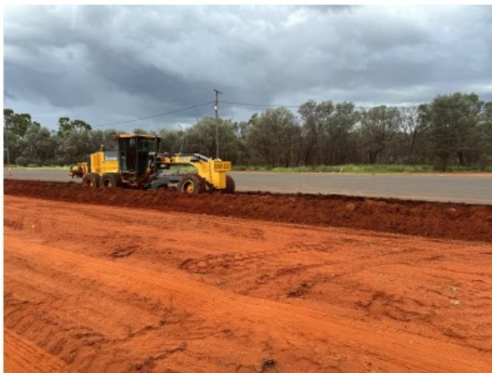
Working at the Charleville Truck Wash site and Slashing of the Landsborough Highway.
