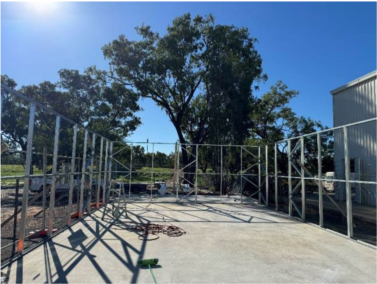
Framing started on the Public Records Shed at the back of the Council Office (W4QLD funded project)
