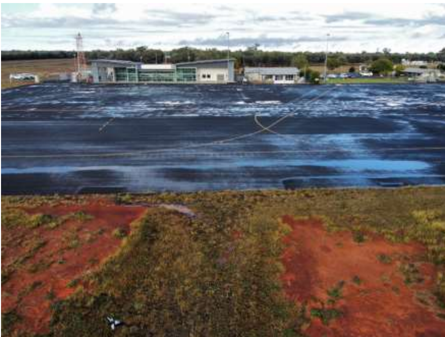
Water pooling on the apron – area in front of the Terminal building
