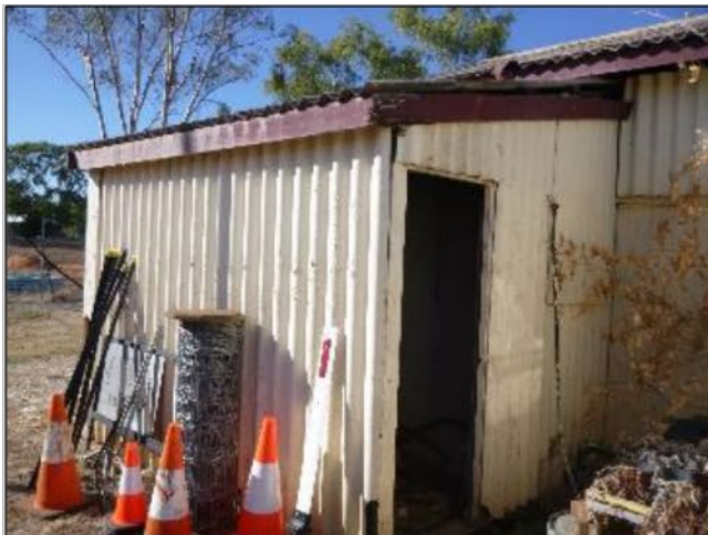
Small side storage room, unpainted roof & damaged walls.
