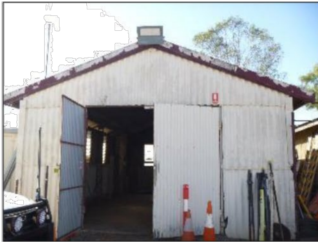
Peeling paint on front roof edge capping.
