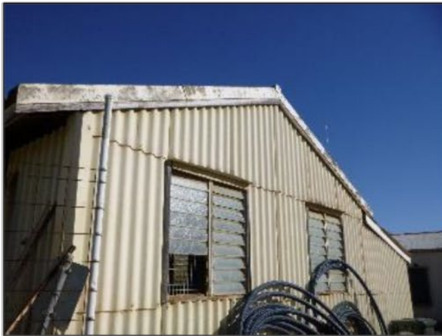
Rear of building, peeling paint on roof edge capping.
