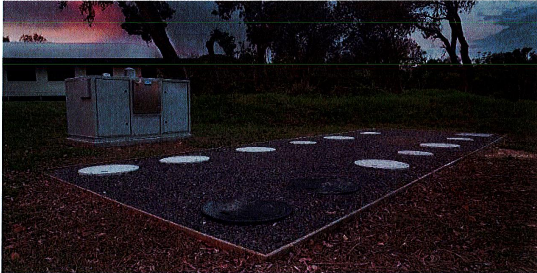
Figure 3-6 Example of installed anaerobic moving bed filter
