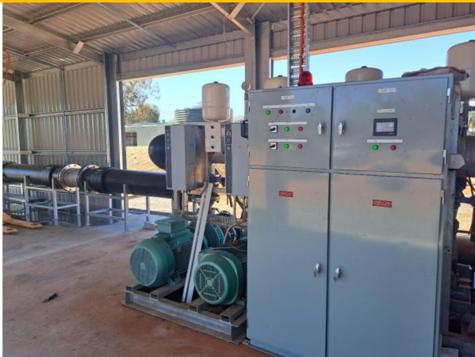
Bore #5 facility has recently undergone an extensive maintenance program and water supply safety upgrade
