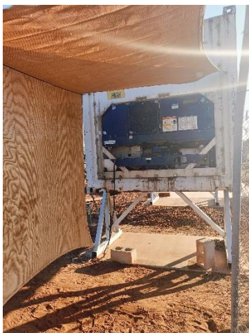
Cover over the cold room motor
